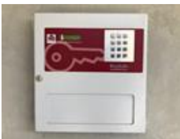
Key Safe Box – located to the left of the Reception window on the entry ramp.
